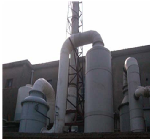
Fig.5 The beryllium-contained waste gas disposal system with a processing capacity of 10 000 m 3 /h
