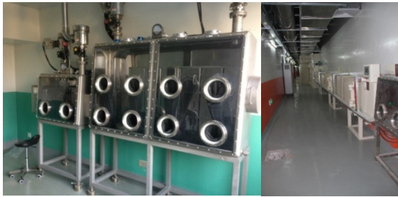
Fig.1 The main process equipment of radiochemical laboratory in building 103
