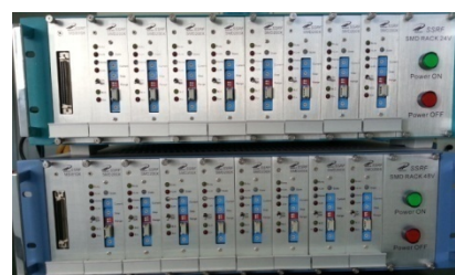
Fig.2 Motor driver and power rack.
